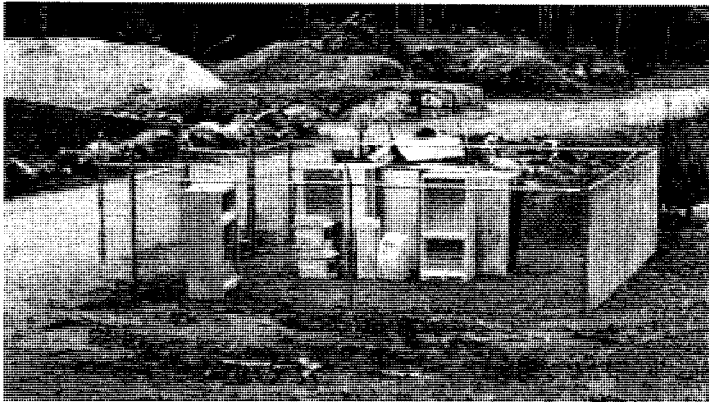
Due to DES regulations which require Freon containing appliances to be protected from vandalism causing gases to be released, we erected a new enclosure.
